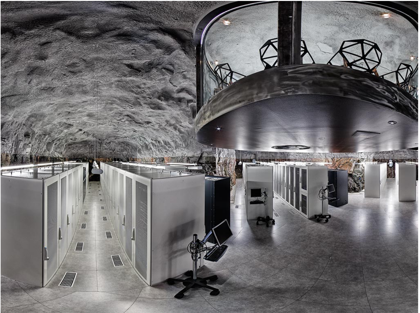
Figure 7. Pionen Datacenter, Stockholm Sweden ( http://i.dailymail.co.uk/i/pix/2010/12/09/article-1337014-0C685E1B000005DC-868_634x419.jpg )
